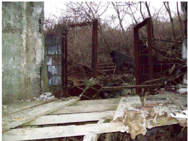
Photo E.22 – View looking into the former Bunker #12 in PAOI 1. Note: The bunker had completely collapsed and conditions were unsafe to enter.
